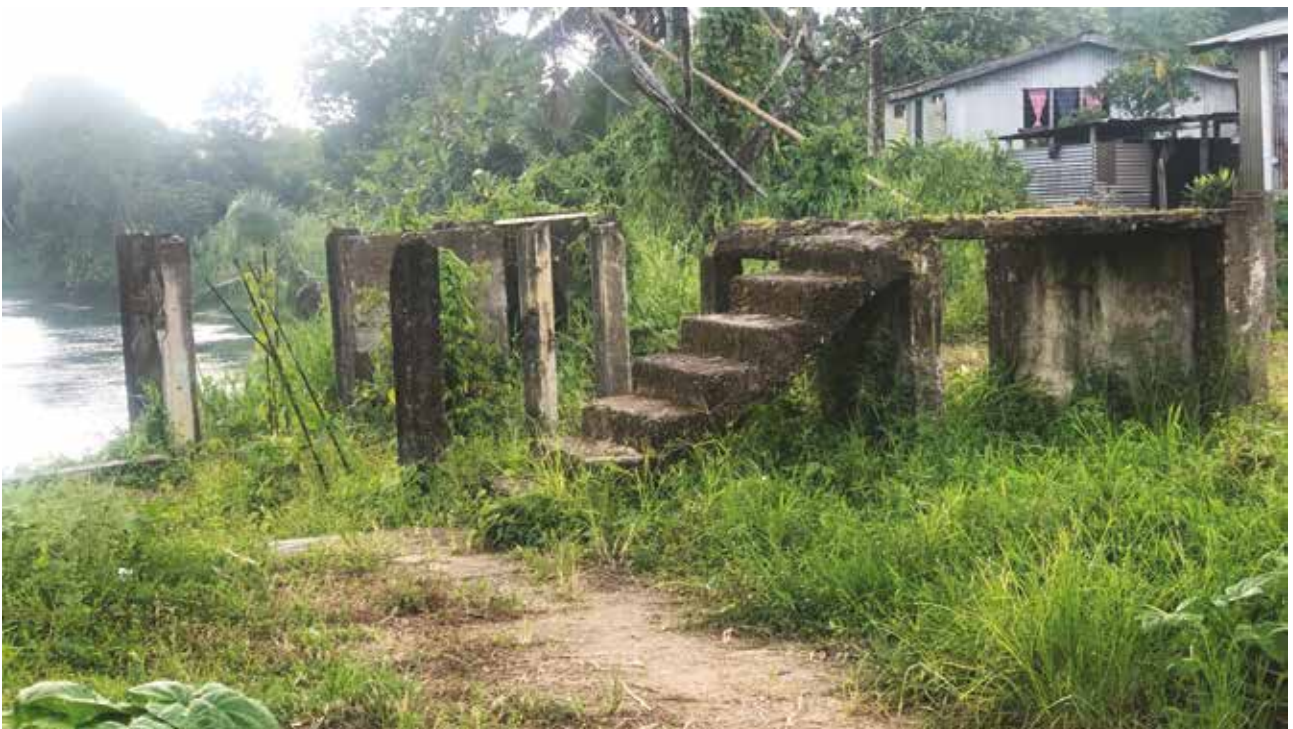
House foundations after flooding at Vuniniudrovu Village. Source: UNITAR
